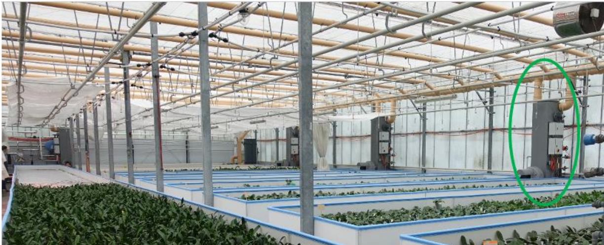
Figure 1: Greenhouse No. 12 of Meyer Orchideen AG. One of the 9 absorbers in market in green (right). The orange pipes on the top are the air suction pipe system. The new structure of table is visible (white wall with blue edge around the crops)
