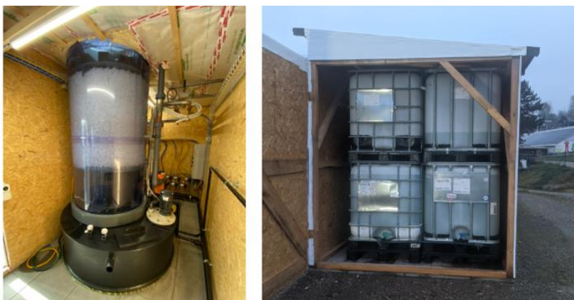
Figure 2: Desorber (left) and TCF storage tanks (right) in the container outside the greenhouse.
