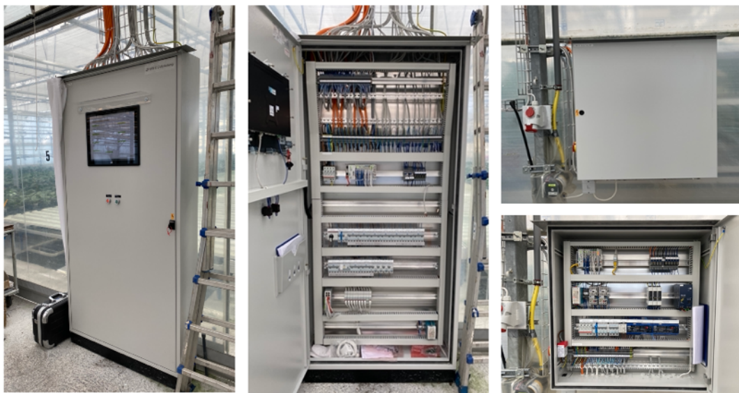
Figure 17: Master Control Cabinet (left, middle) and Absorber Control Cabinet (right)
