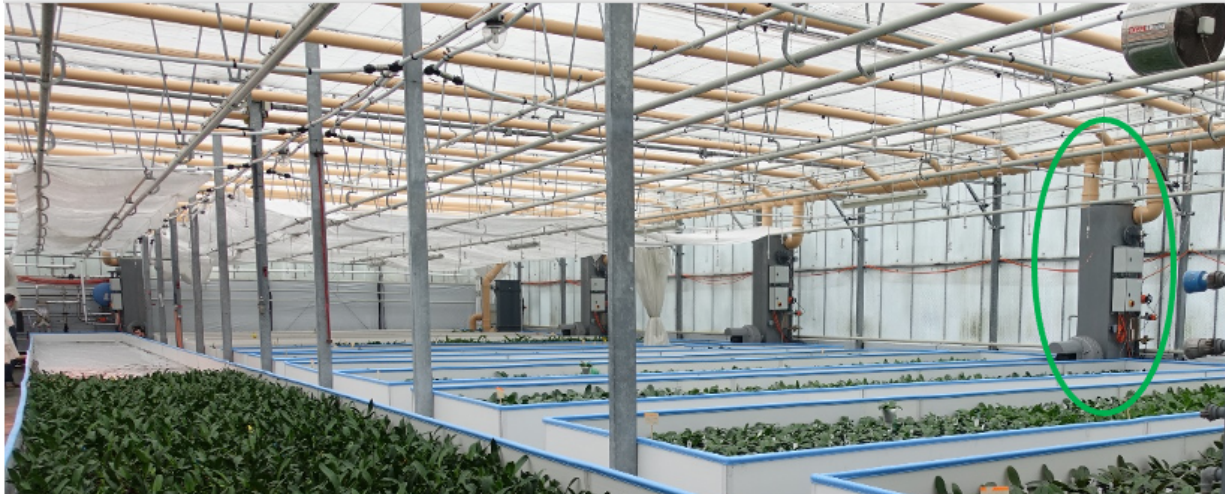
Figure 5: Greenhouse No. 12 of Meyer Orchideen AG. One of the 9 absorbers in market in green (right). The orange pipes on the top are the air suction pipe system. The new structure of table is visible (white wall with blue edge around the crops)
