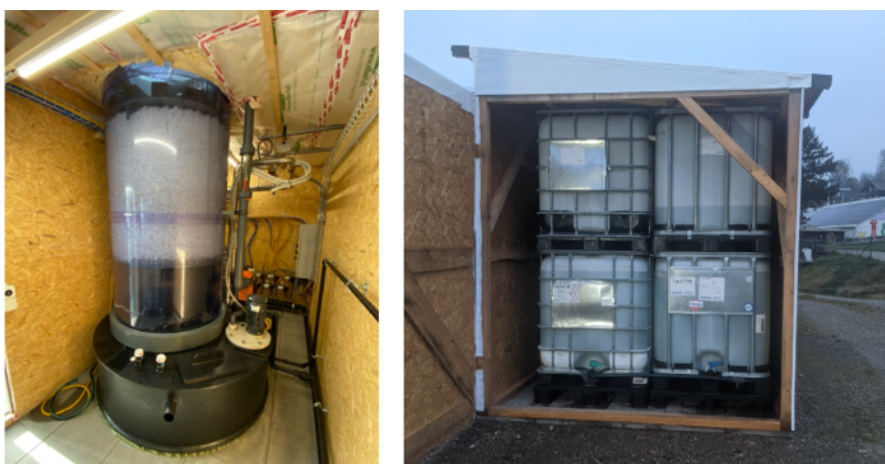
Figure 6: Desorber (left) and TCF storage tanks (right) in the container outside the greenhouse.
