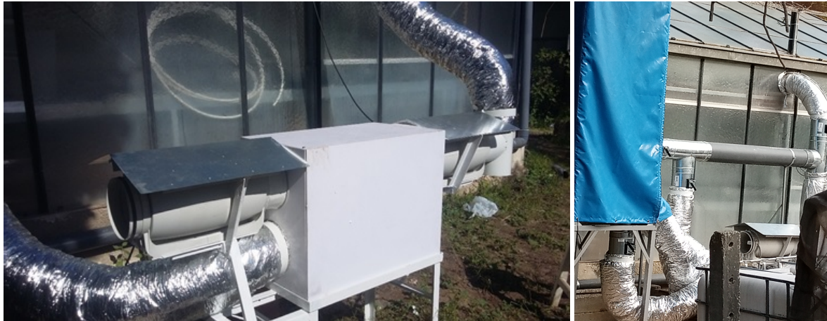
Fig.13-14 Air to air heat exchanger and Watergy absorber, integrated in air distribution network
