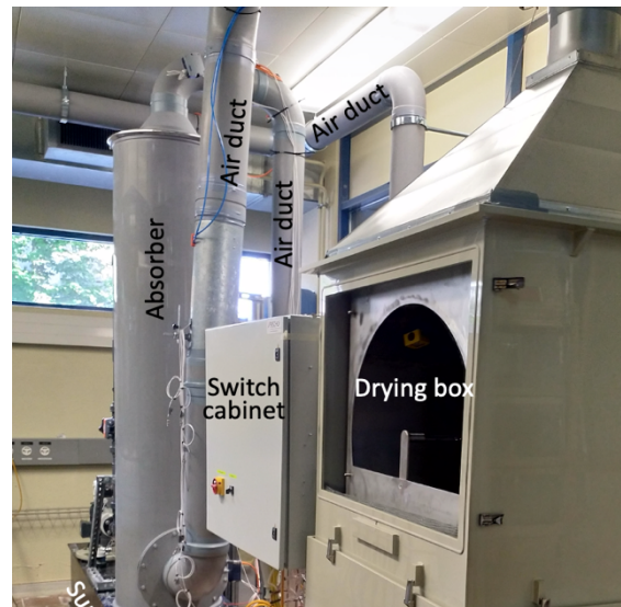
Figure 4: the demonstration plant at the ZHAW used for TheGreefa project
