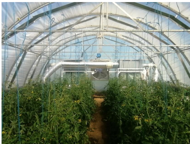
Figure 1. The Liquid-Desiccant Air-conditioning System installed at TheGreefa Tunisian demonstrator
