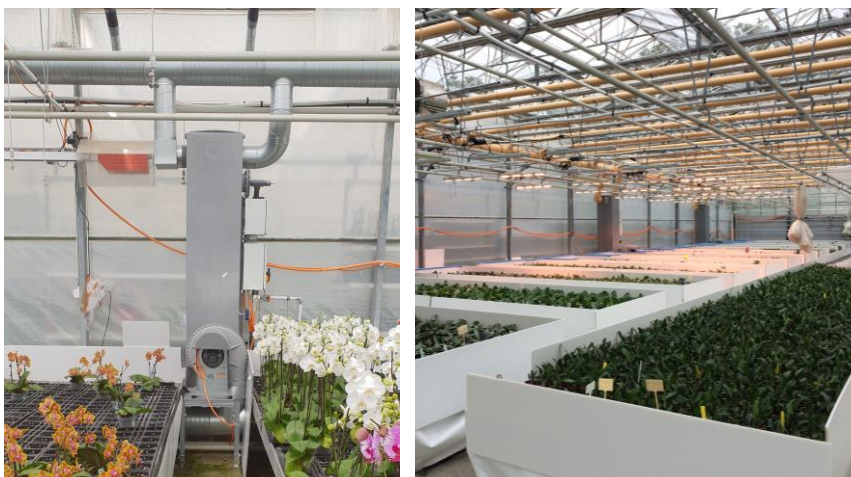
Figure 53. The absorber unit (left) and planting tables (right) in the greenhouse in Switzerland.
