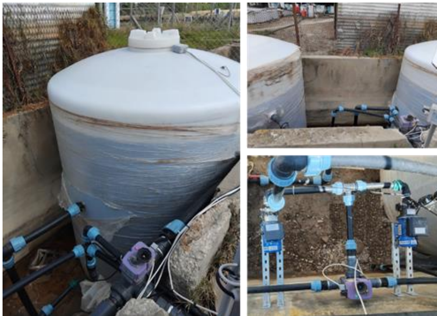
Figure 34. Pumps and electrovalves.
