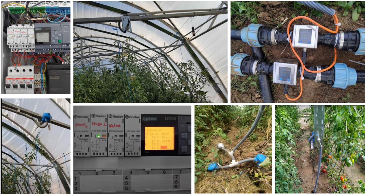
Figure 36. Installation of the control box, the sensors and the data acquisition system.
