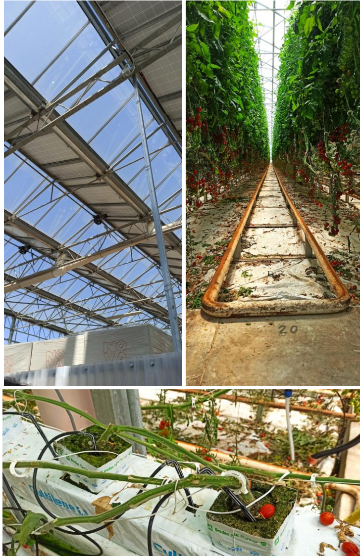
Figure 54. Sfera Agricola’s greenhouse – roof system (top left), piping heating system (top right) and the tomato plants with sensors (bottom).
