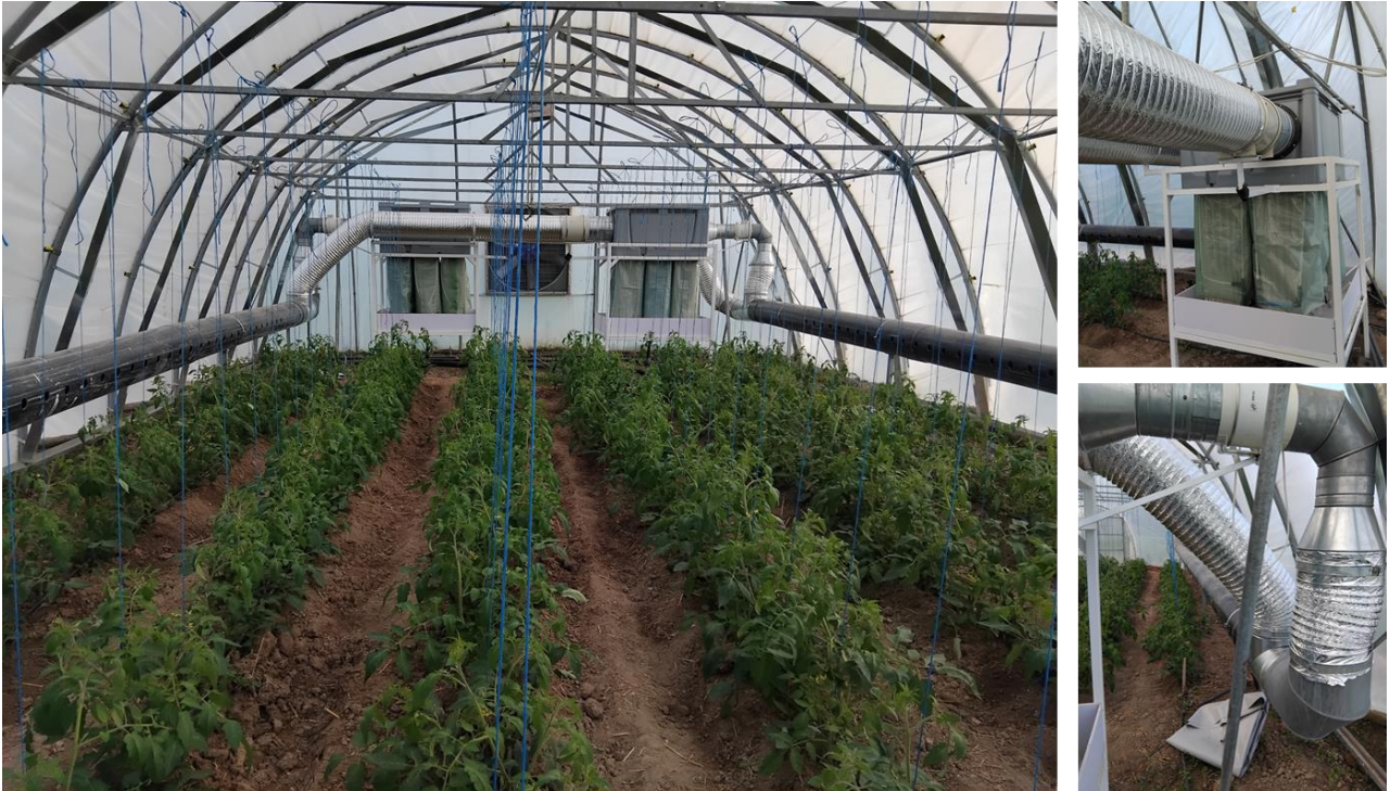
Figure 35. Installation of the Absorber devices and the air circulation system inside the greenhouse (fans + air ducts).
